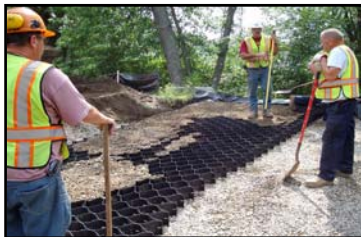
L to R: Tim Schanz, Jim Kiernan and Dave Hobert repairing Prescott Bridge
